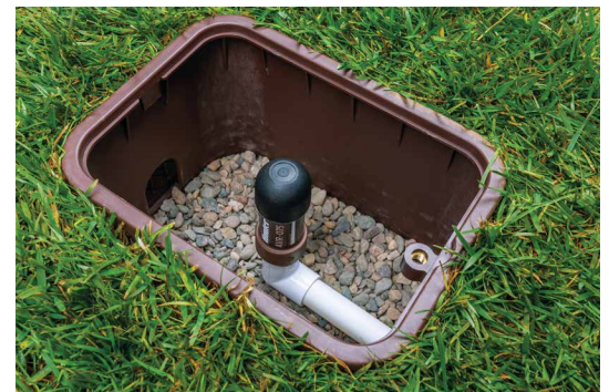
Air/Vacuum Relief Valve Installed
