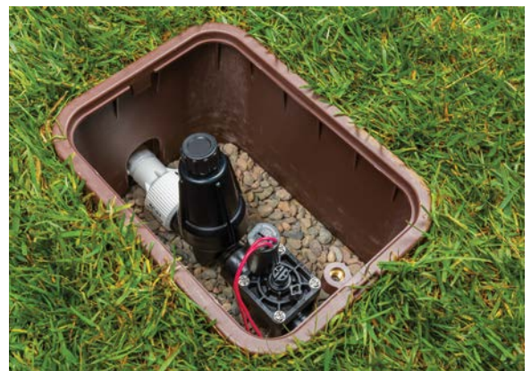
PCZ-101 installed in a Multi-Purpose Box
